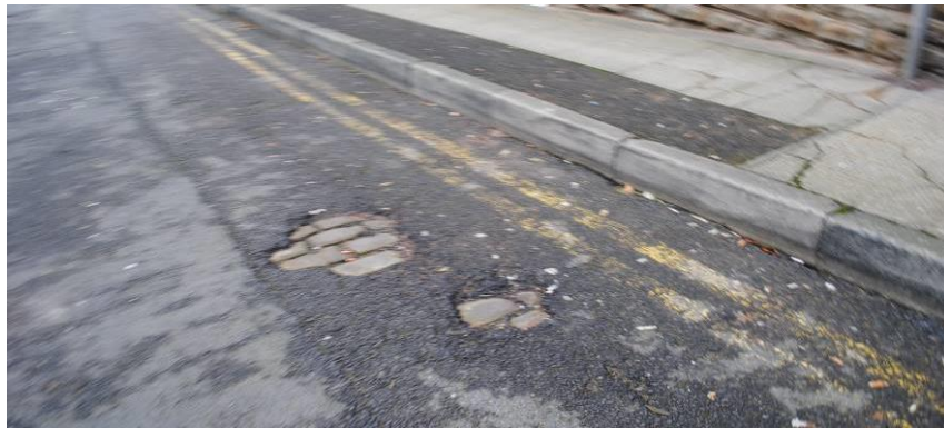
Figure 72 Failed street surfaces on Parish Street
