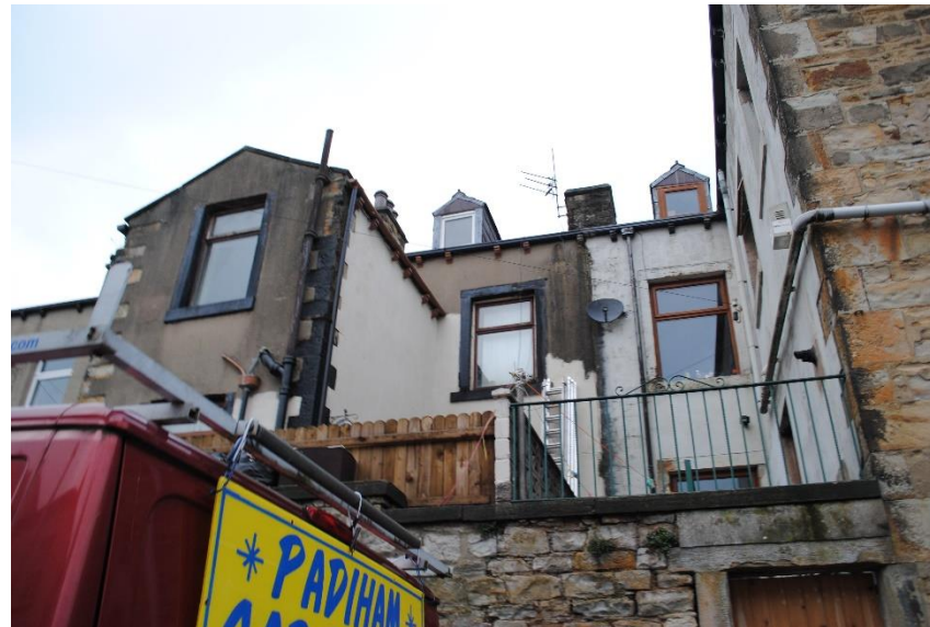
Figure 52 Queen Street: example of condition
