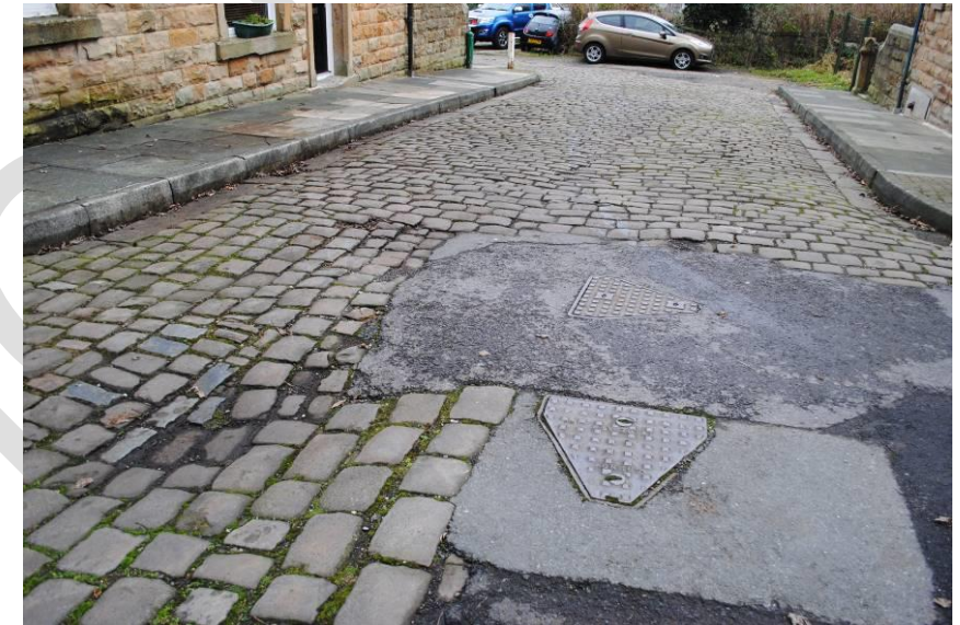
Figure 58 Poor quality surface repair on the corner of Dragon Street and Albert Street.
