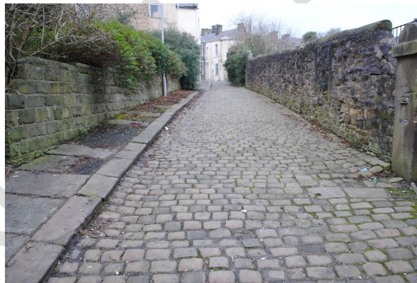
Figure 25 Tarmac on Church Lane footpaths
