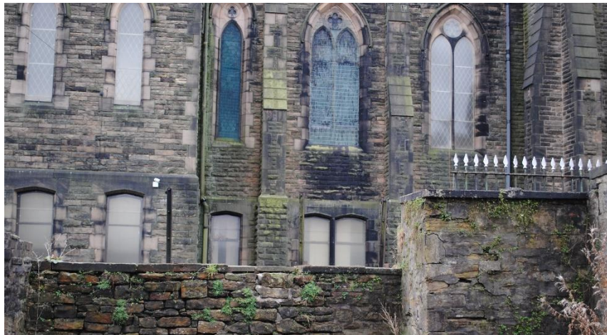
Figure 77 Detail of Unitarian Chapel showing blocked windows, vegetation growth and evidence of water ingress.
